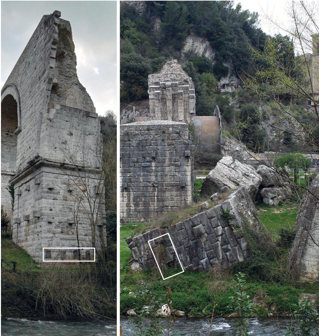
Figure 8. Holes in first and second pylon.
