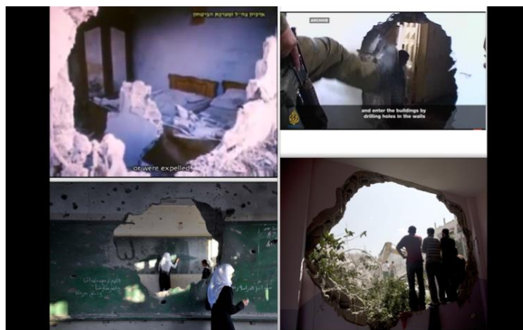
Figure 5 - Images board, damaged walls. Photo credits from upper left to right clockwise: Looted and Hidden, film still; Rebel Architecture, film still; Middle East Monitor; Mahmoud Hams/AFP)
