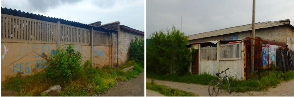
Figure 5.4. Large concrete barriers served to wall factories and other state facilities off from the rest of the built environment. These are seldom removed despite the end of state control and central planning. Source: Baialieva, Shamaldy-Sai bazaar, 2018.
