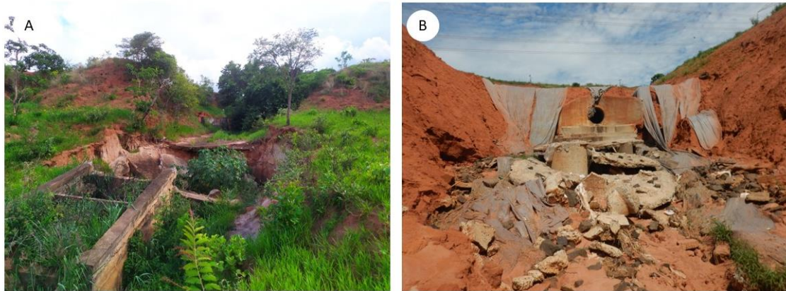
Figure 13. Erosion containment structures damaged by lack of maintenance or sizing errors: a) Jardim Grama; and b) Quinta da Bela Olinda.
