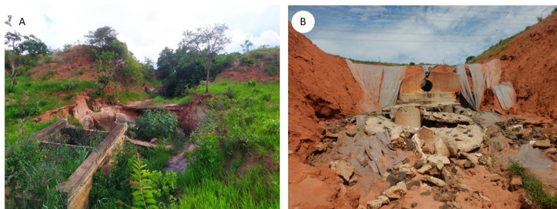
Figure 4. Erosion containment structures damaged by lack of maintenance or sizing errors: a) Jardim Grama; and b) Quinta da Bela Olinda.
