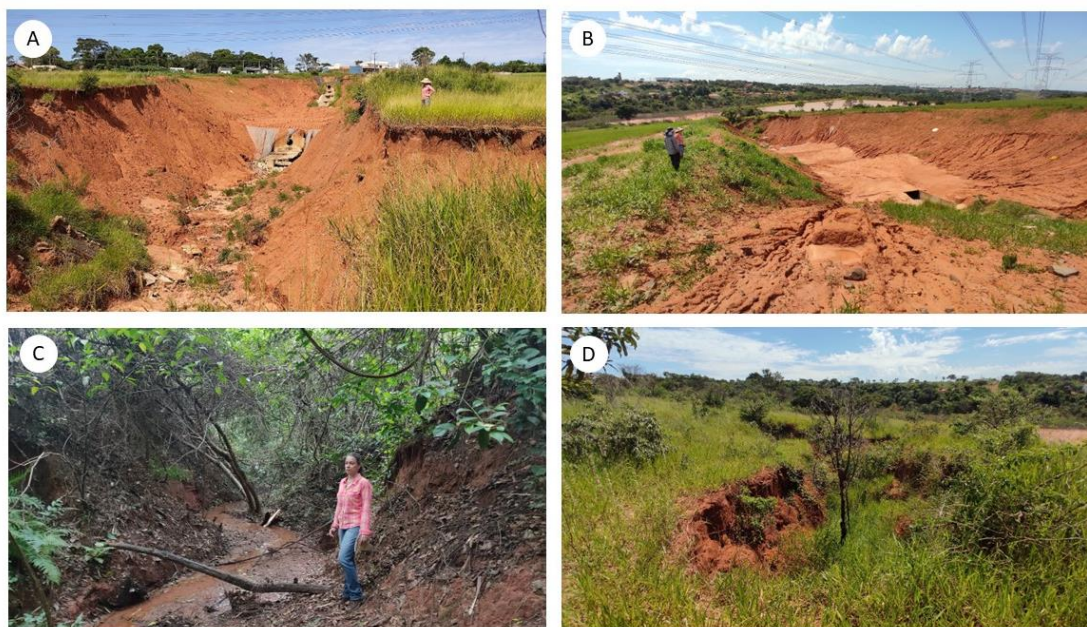
Figure 7: a) top view of ravine 5, the implemented works already have some of their functionality damaged, b) top view of ravine 5, where it is possible to observe grooves demonstrating the concentration of surface runoff into the ravine channel; c) gully 1, which shows water flow in the channel and vegetation composed of trees in the surroundings; d) ravine 2, with pasture and small trees inside and around the channel, indicating stability of the feature.
