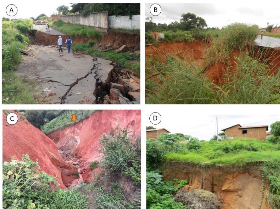
Figure 4. Examples of gullies and ravines in Brazil. A and B: Gully located at Rua 14-E, municipality of Aparecida de Goiânia, state of Goiás (Cardoso 2013); C: Unstable areas with imminent risk of landslide. Santana do Mundaú, state of Alagoas (Da Silva 2018); D: Ravine under development, 3 meters from residences, municipality of Timon, state of Maranhão (De Oliveira Filho and Dos Santos 2014) (Source: S2ID system reports).
