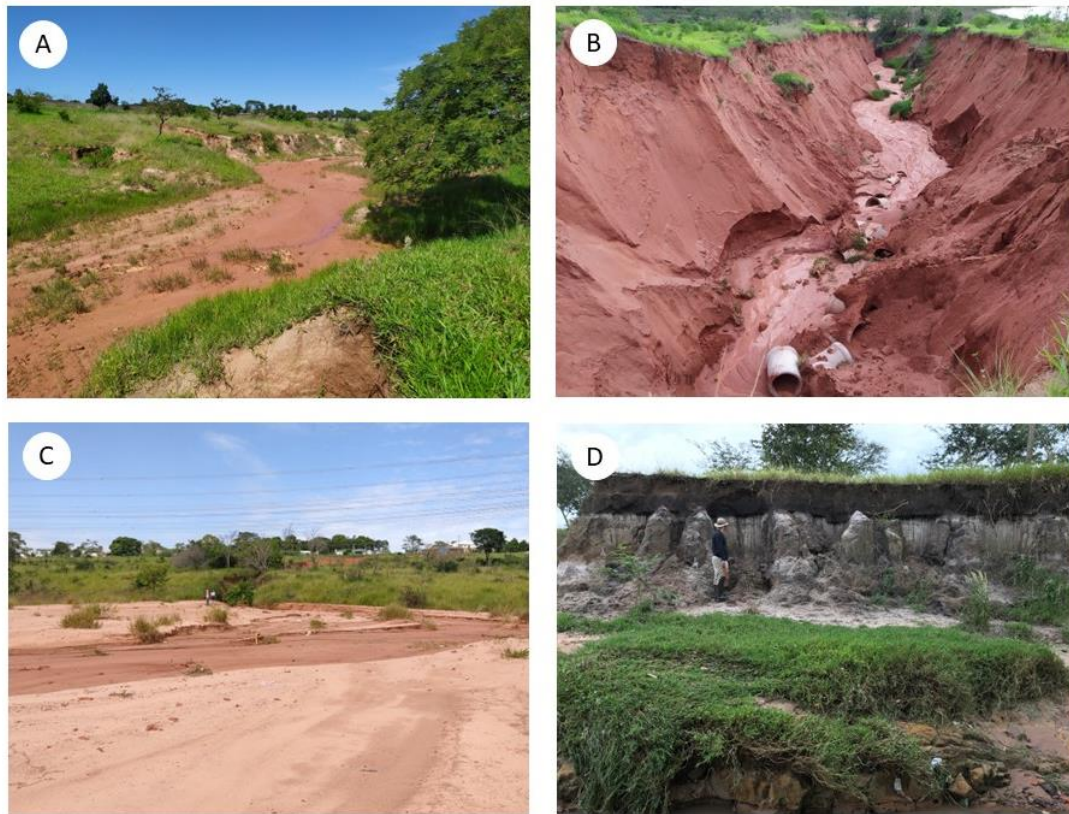
Figure 12. A) Erosion process at the valley bottom, where the lowering of the channel upstream and the silting and drying of wetlands downstream occur; B) ravine at Quinta da Bela Olinda, developed due to problems in stormwater sewers; C) silted-up area in the region of Quinta da Bela Olinda; D) soil profile, indicating lowering of the channel and drying of wetlands.
