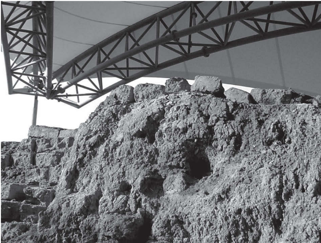
Fig. 9 Under the G6 roof; the original Troy II mud- bricks are protected with a layer of specially created »burned« brick – the formula is included in the Appen- dices. Provided by the author.
